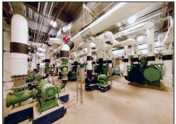
The mechanical room for the pumps and water chillers, located on the lower level of the Great Hall.
